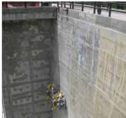
Kryton's Krystol Crack Repair System was used to repair leaks in the dam face.
